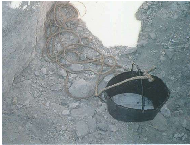
Figure 8c: Bucket to be filled with excavated material and hoisted to the surface on a rope.
